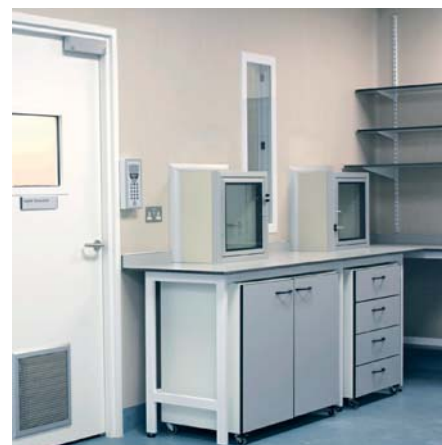
The assembly room, part of the newly-built clean room, designed so that pressure differentials run from rooms of high to low classification
